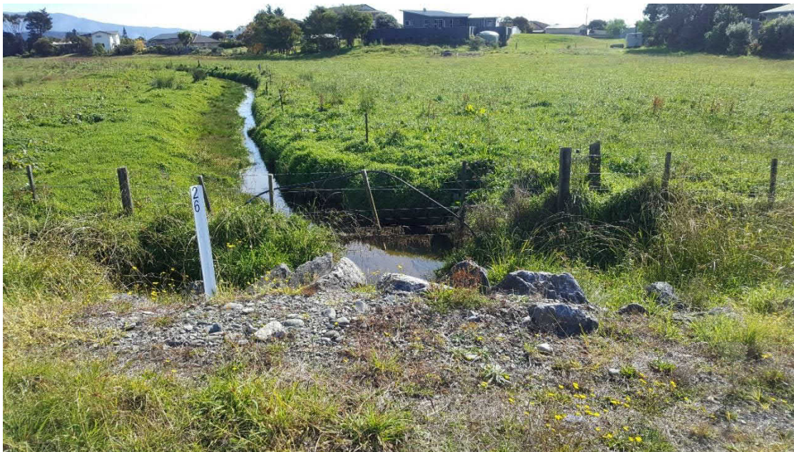
Figure 2.5: Bartlett Creek looking downstream from outlet of existing Abel Tasman Drive culvert. Location of Bartlett Creek bund (west) can be seen at right hand side of photograph.
