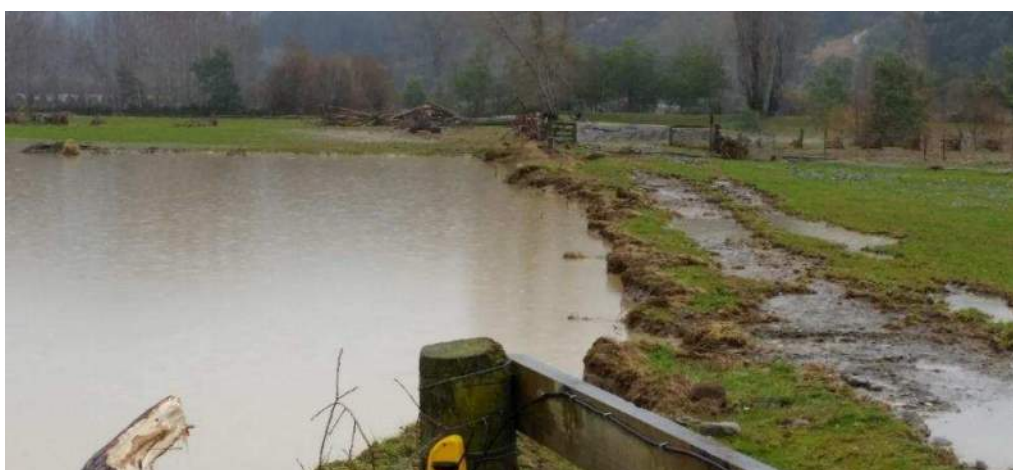
Figure 6b: CJI Ltd gravel extraction to the boundary plus erosion of neighbouring boundary. Photo taken 18.7.21.
