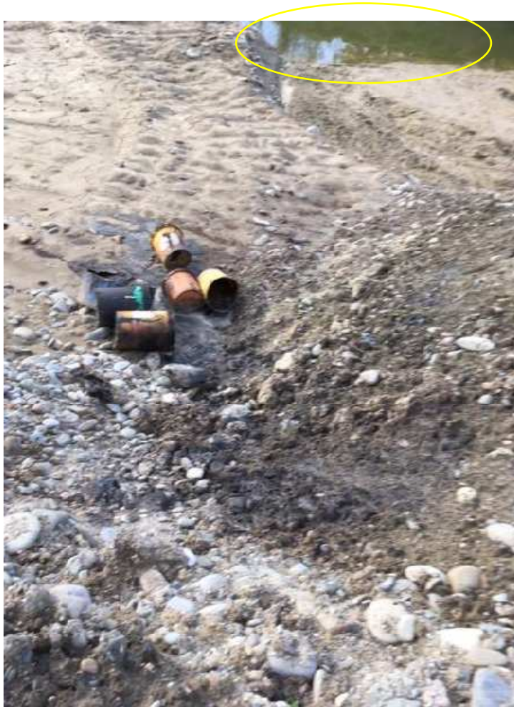
Figure 5: Oil drums and standing water in Douglas Rd gravel pit-Back-fill. Photo taken 23.8.21.
