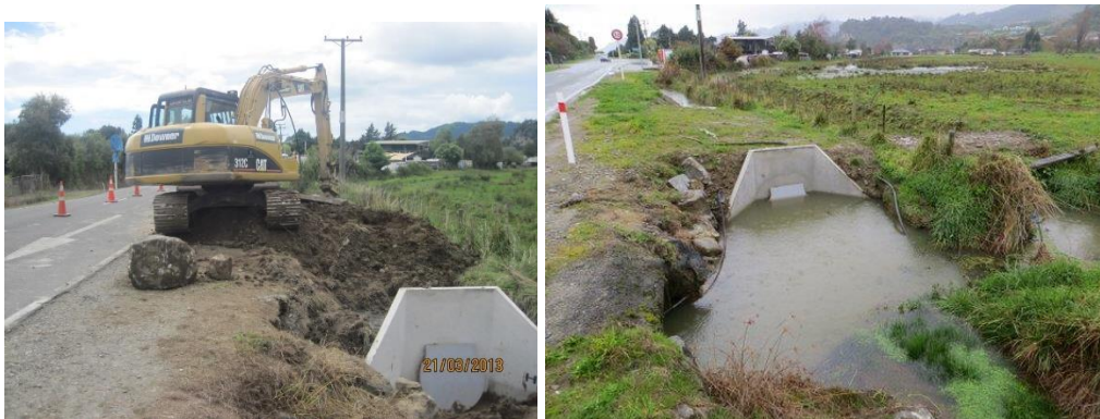
Photos 6, 7: Installation of flap gated culvert just south of 734 Abel Tasman Drive (March 2013, left) and operation in rainfall event (June 2013, right)
