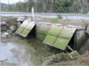
Causeway with tidal flapgates - Motupipi Inlet
