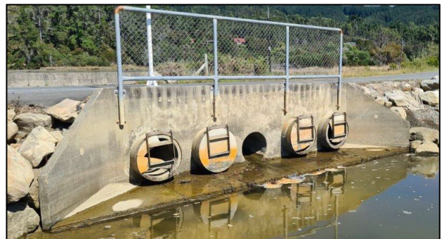
Culverts at mid-outgoing tide on main estuary side (bottom), showing flap gates on the four culverts that are perched above the bed level. Only the central culvert is draining the embayment. The flap gates on the four perched culverts were partially closed and/or broken.
