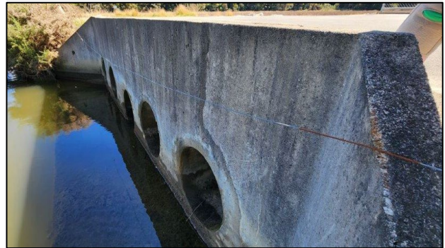
Culverts from embayment side (top and middle), with only one flowing during the mid-outgoing tide.
