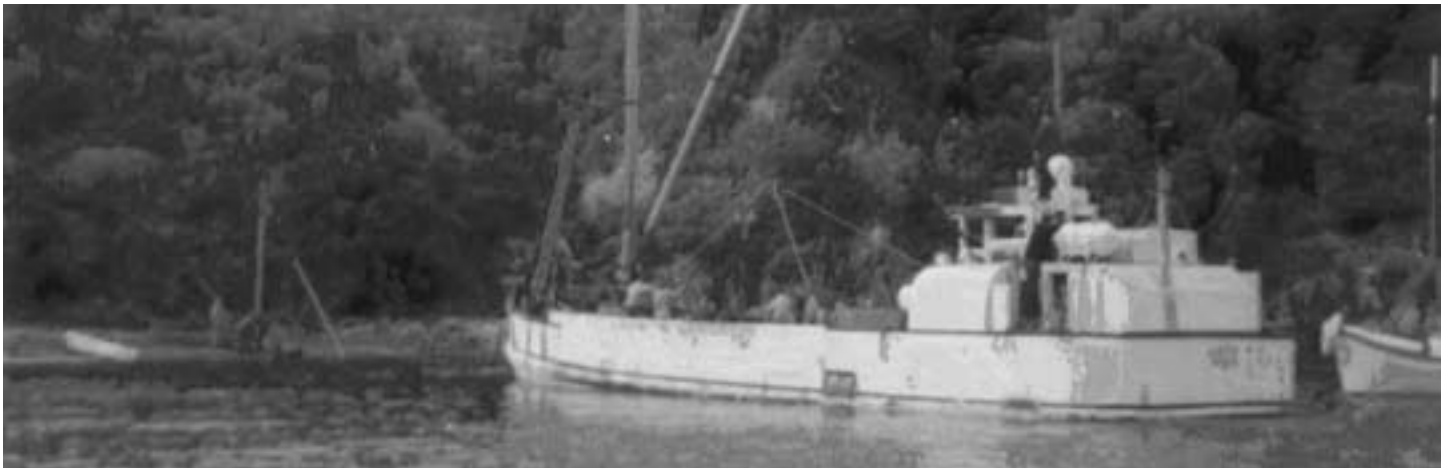
The Vesper lays the telephone cable between D'Urville Island and French Pass.
