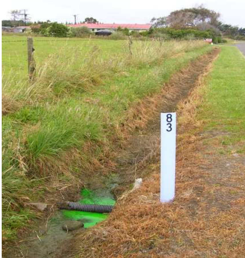
Dye discharge: piped from domestic tank to roadside drain; then discharges through culvert 83 onto a Golden Bay beach.
