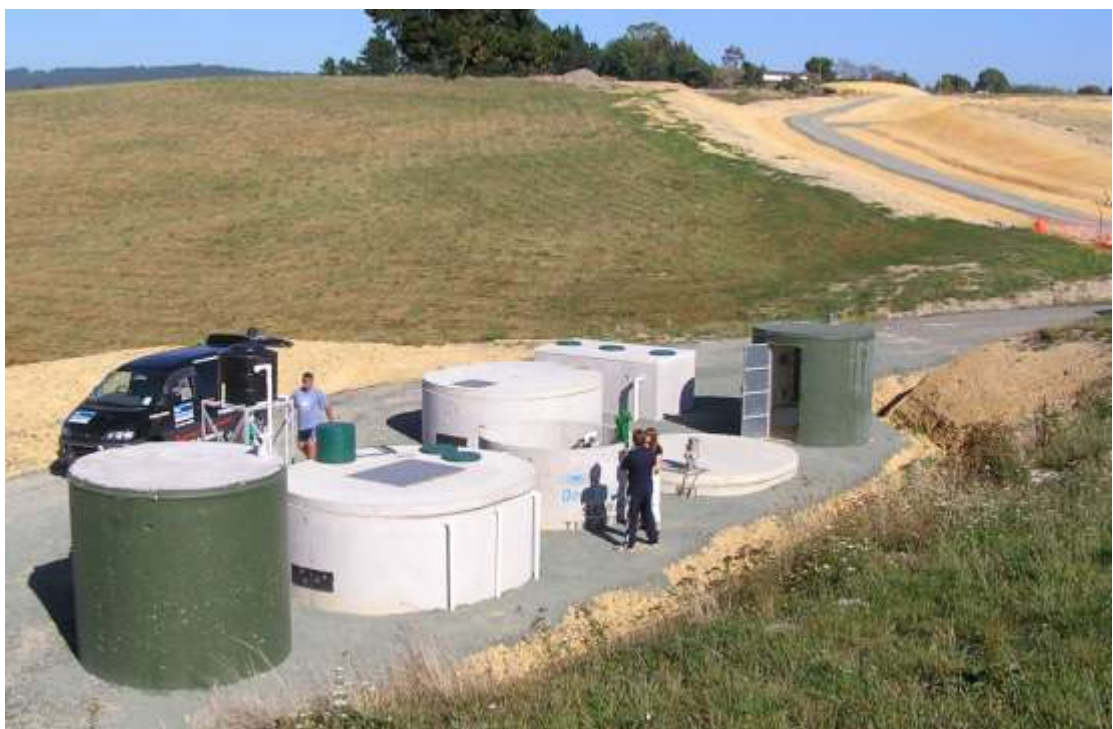
Privately owned cluster system installed to service a new subdivision
