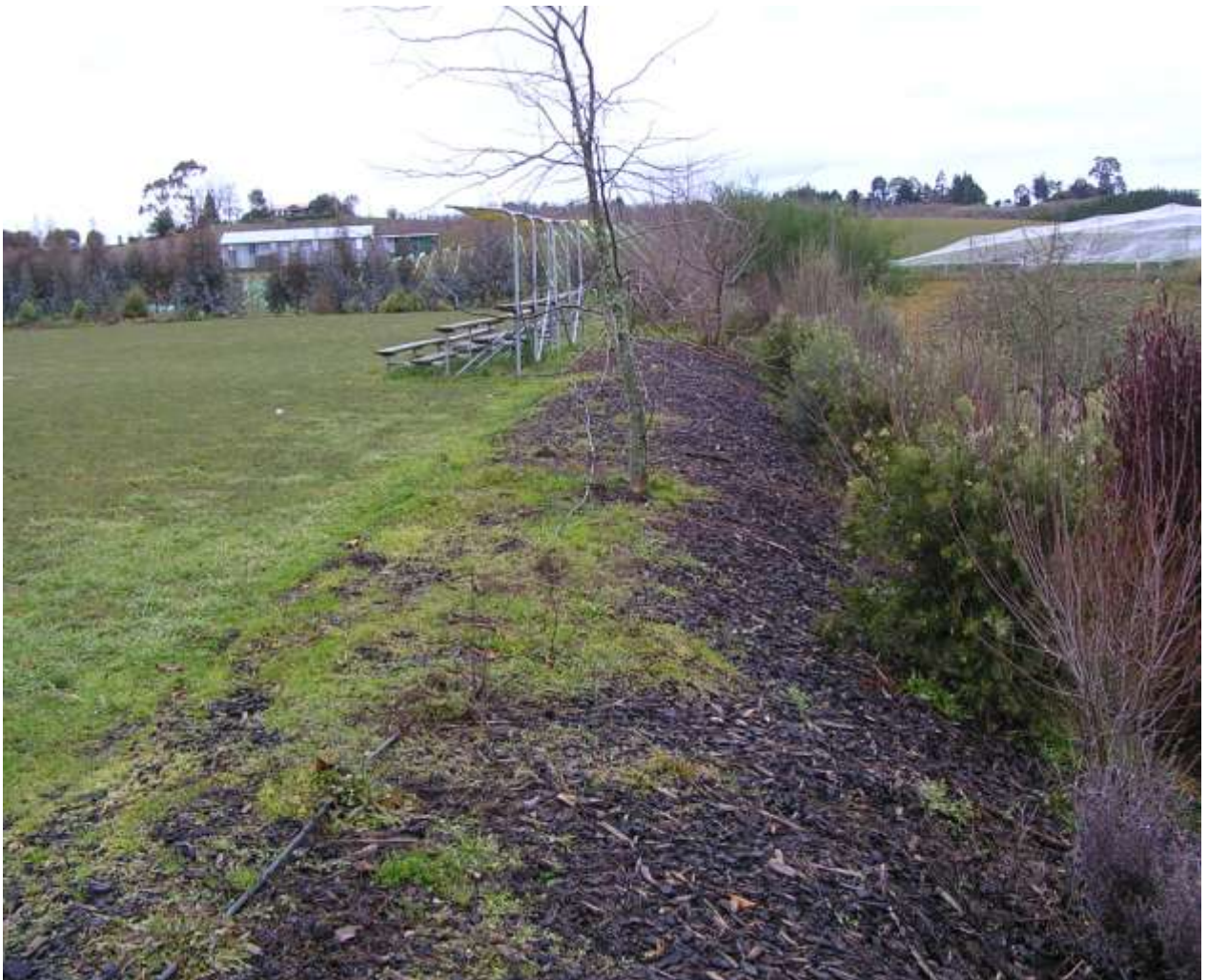
Note the black pipe running alongside the school playground in an area where children play. This is a wastewater disposal pipe cut in places by a lawn mower and discharging secondary treated sewage from the school on-site wastewater treatment plant directly onto the playing field.
