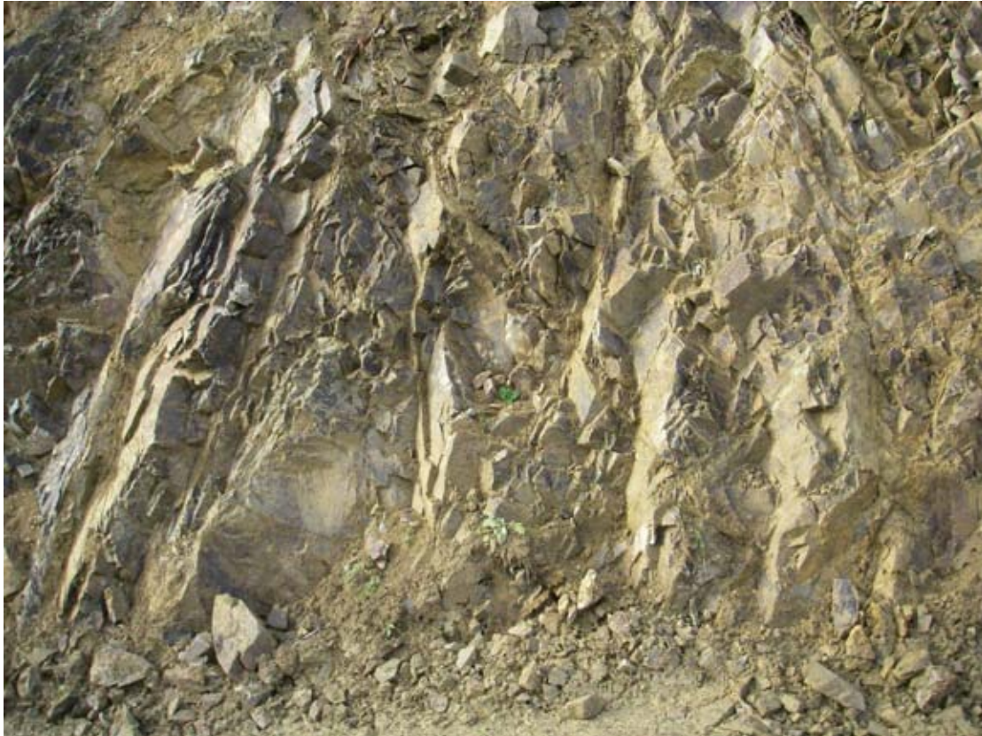
Photo 11: Moderately weathered, closely jointed rock exposed in track upslope of right abutment
