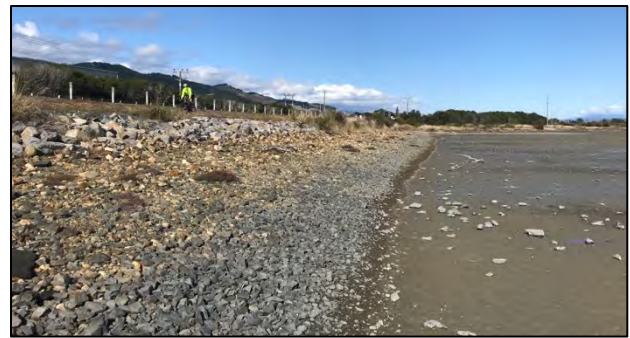
Artificial rip-rap and cobble protection adjacent to the cycle lane and Whakatu Drive
