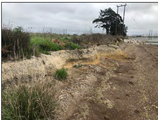
Eroding shoreline (foreground) and rock rip-rap protecting power poles in the background west of Reservoir Creek.
