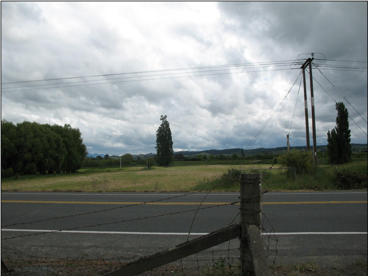
Electricity transmission lines at Appleby Bridge
