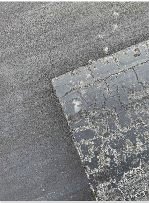
Blasting, chipping fading or obscurity due to rubber build up:
