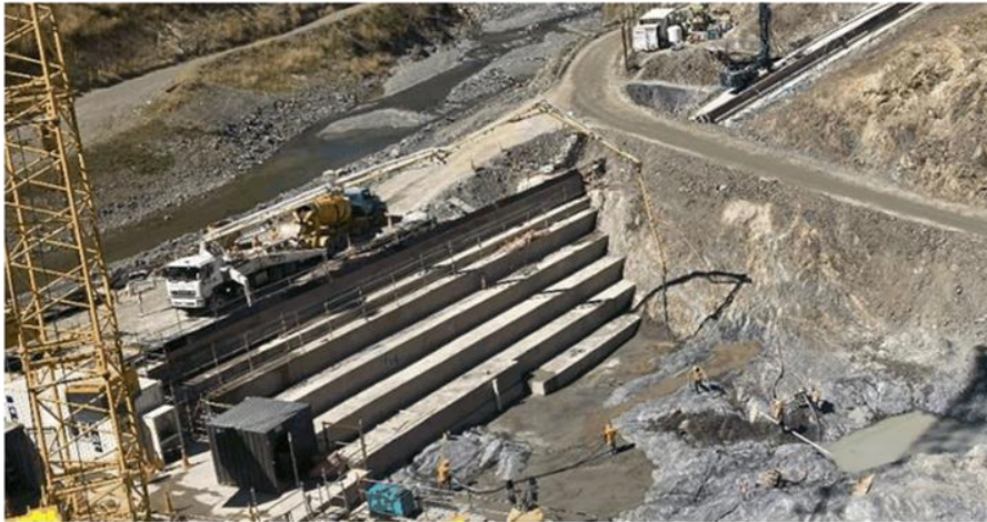
Figure 38: Pouring mass concrete at embankment foundation defect area immediate downstream of starter dam, Feb 2021
