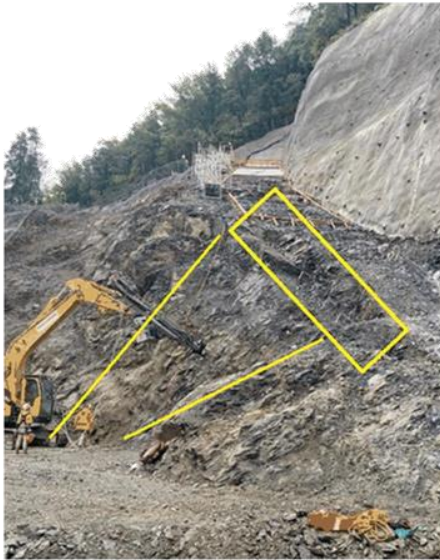
Figure 39: Deficient foundation rock
