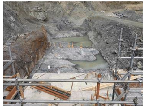
Figure 37: Voids to be treated beneath the culvert
