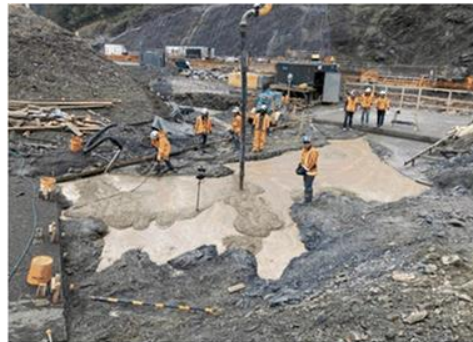
Figure 36: Concrete to voids on the LHS plinth
