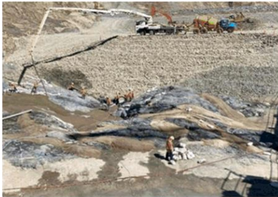
Figure 7: Defect treatment of third Embankment foundation
