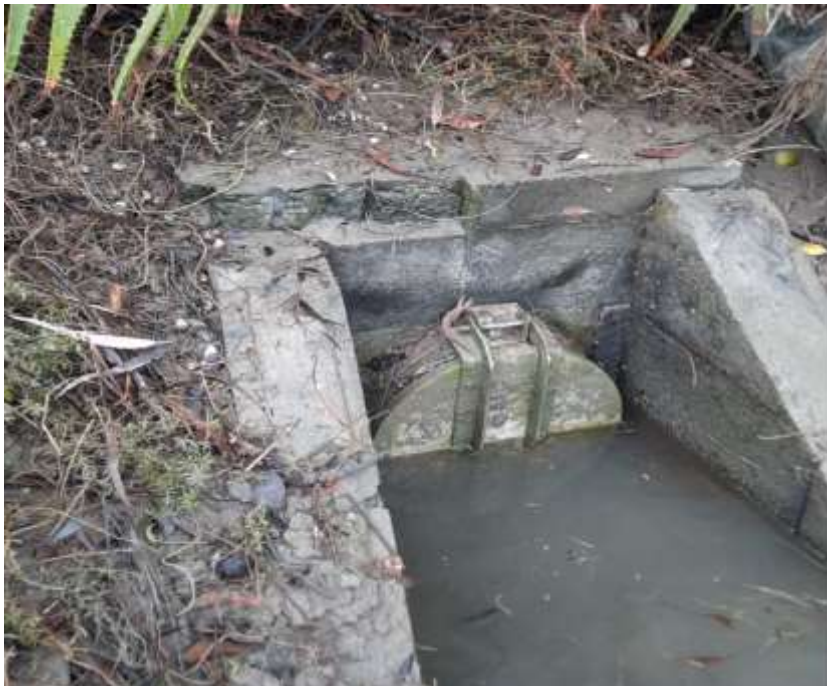
The two in-line floodgates – one upstream in a manhole chamber and the other opening out into the estuary – near Everett Street, Motueka.
