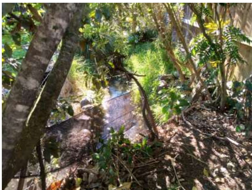
Restrictive pipe outlet location of 600mm diameter pipe - Hill Street, Richmond.
