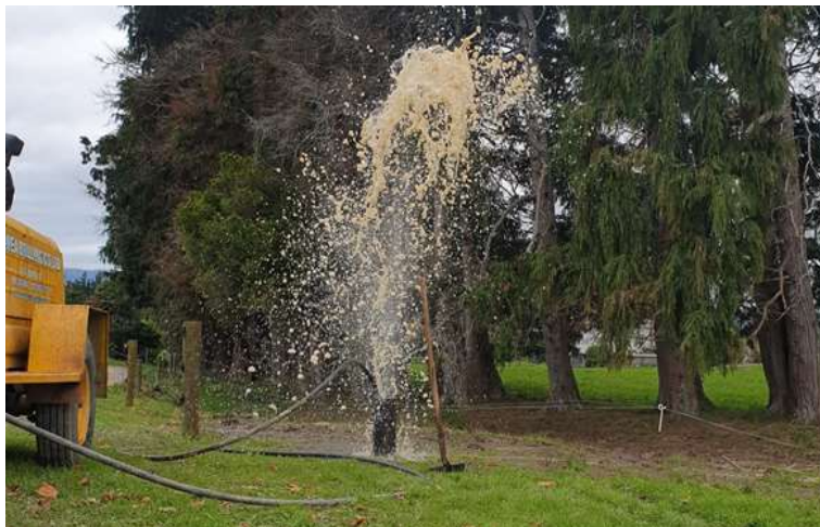
WWD 24432 - Wigzell Road. Photo showing the bore being developed (via air lift) to clear the fine grained sediment from the bore in preparation for the pumped aquifer test.
