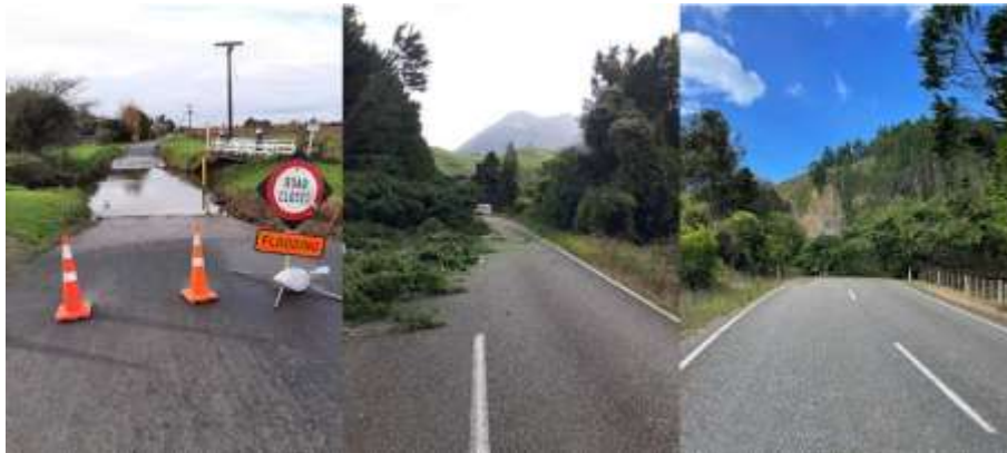
Golden Hills Road ford, and fallen trees on Motueka Valley Highway
