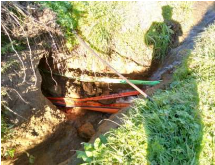
Services trench undermined - Pohutukawa Place, Pohara.
