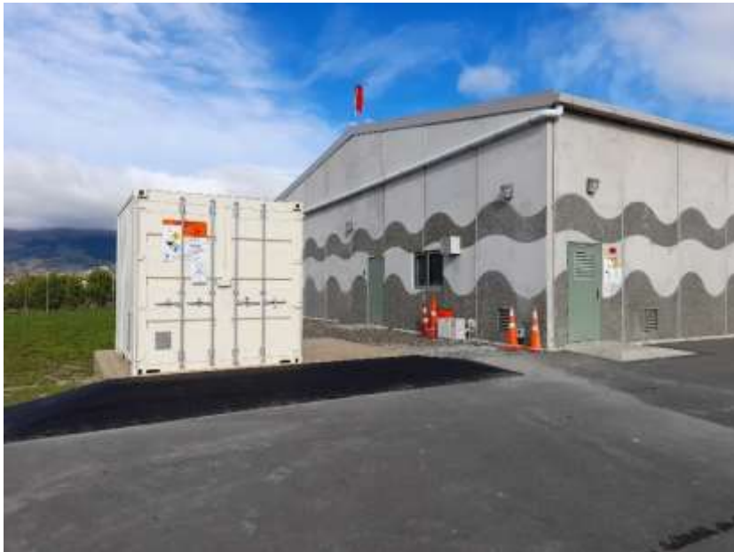
Chlorine storage container, Richmond WTP
