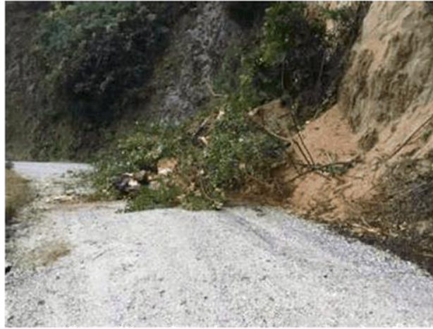
Totaranui Road slip
