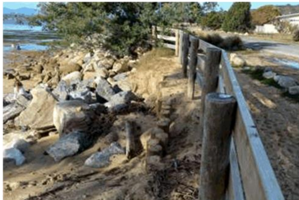
Erosion at northern end of Marahau rock revetment
