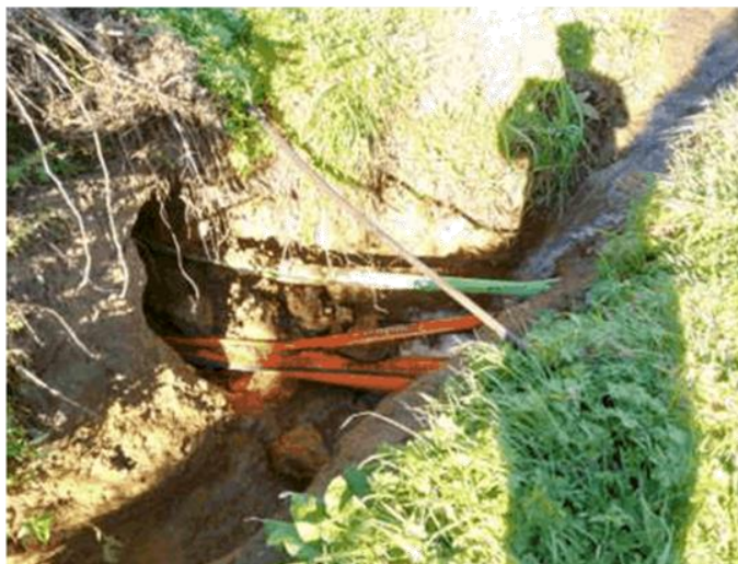
Services trench undermined - Pohutukawa Place, Pohara.
