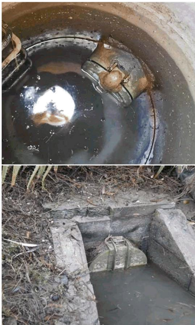
The two in-line floodgates – one upstream in a manhole chamber and the other opening out into the estuary – near Everett Street, Motueka.
