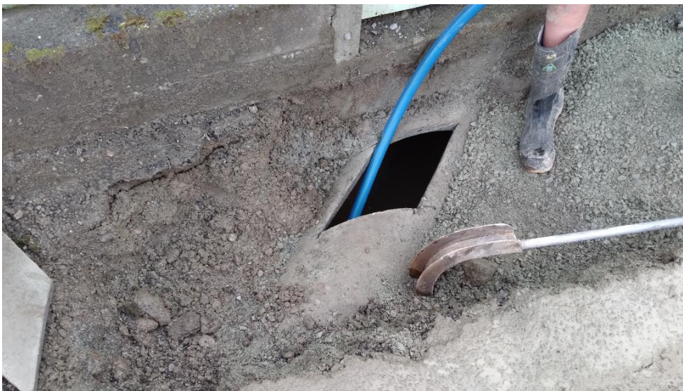
Pipe cut to allow access into pipe for trenchless hydraulic root cutting equipment - Doris Street, Richmond, below Hill Street. Sump to be installed here to allow a permanent access point.
