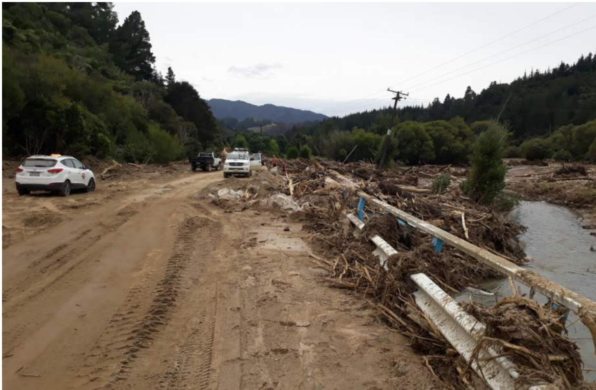
Silt and Debris - Riwaka-Sandy Bay Road
