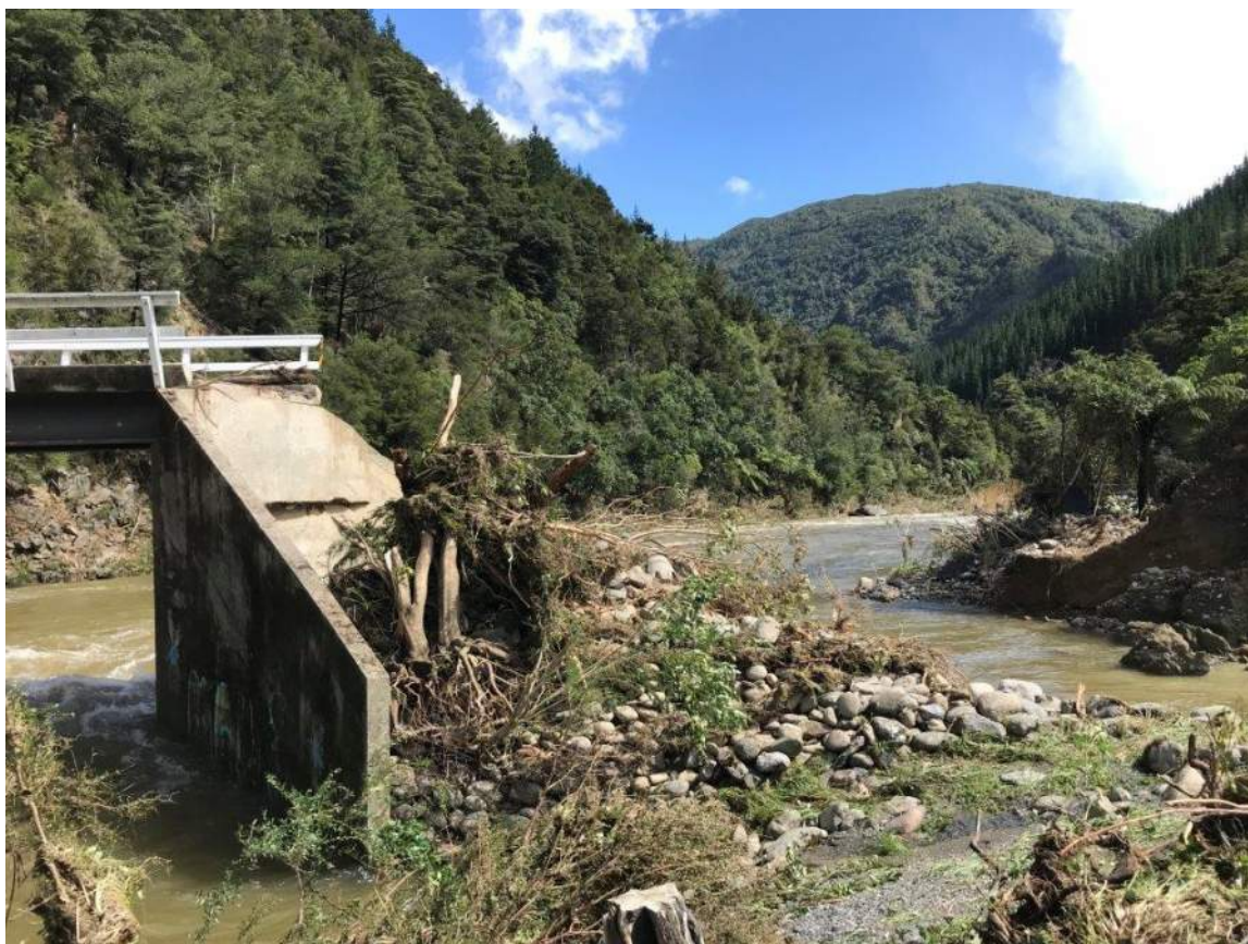
Cobb Valley Bridge approach washed away
