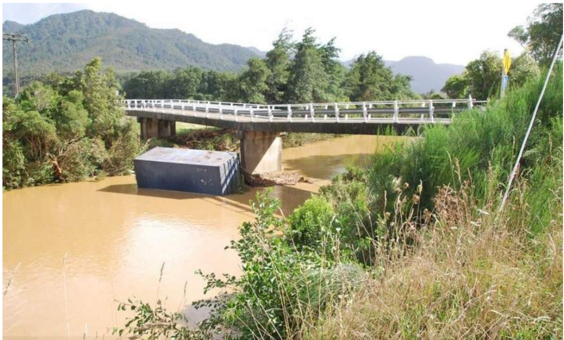
Kaituna Bridge central pier has settled
