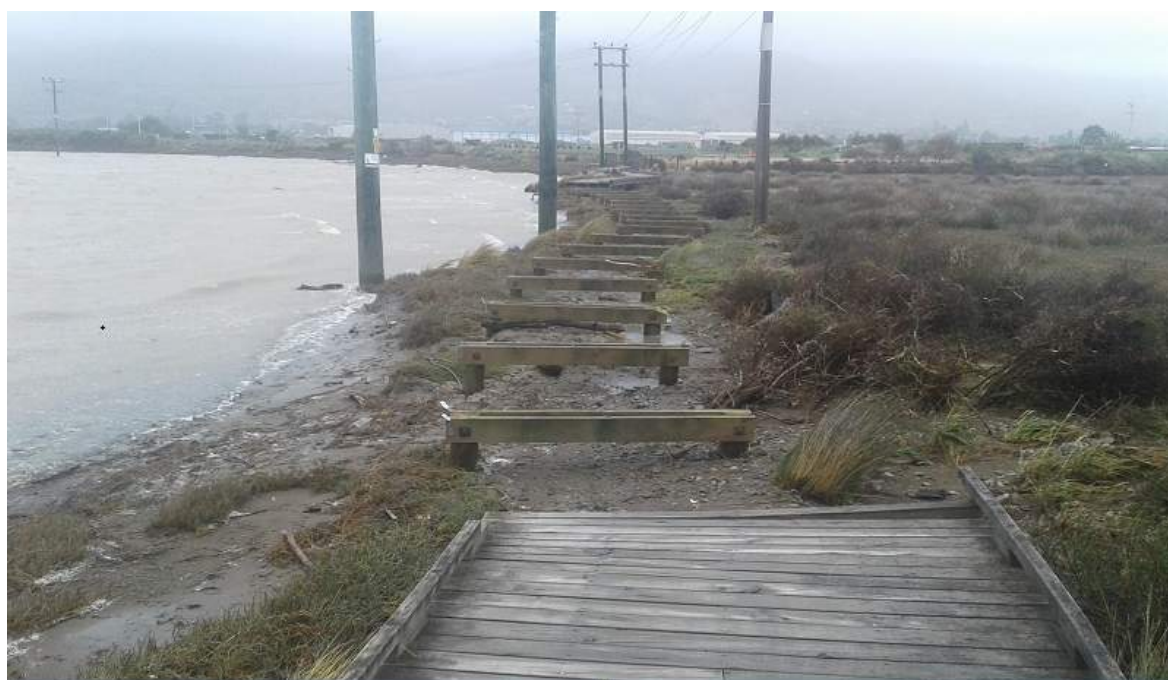
Coastal cycle trail – Boardwalk Damage
