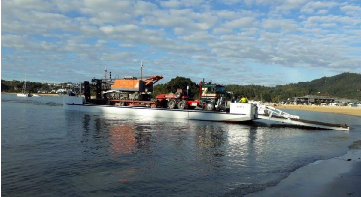
The crawler crane (39 tonne) transported by low-bed transporter (truck and cargo total approx. 65 tonne) loaded onto Barge at Kaiteriteri.
