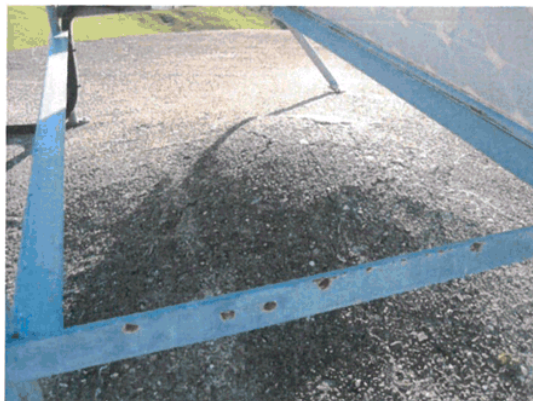
Photo 3-28: Close-up view of damage to roof slab at Silcocks concrete tank – Dovedale.
