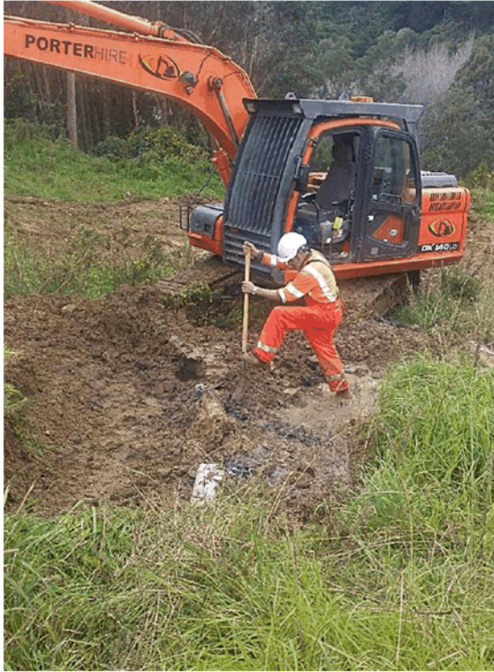
Figure 8.10 Men at work dealing with a leachate outbreak in 2014
