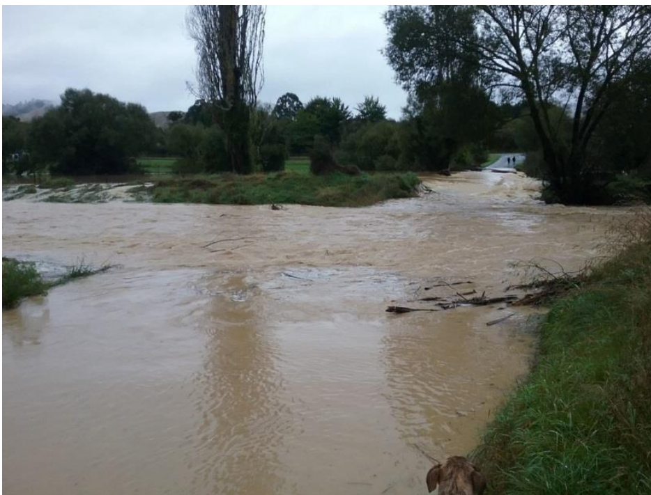
Flood waters across the Thorn Road concrete splash
