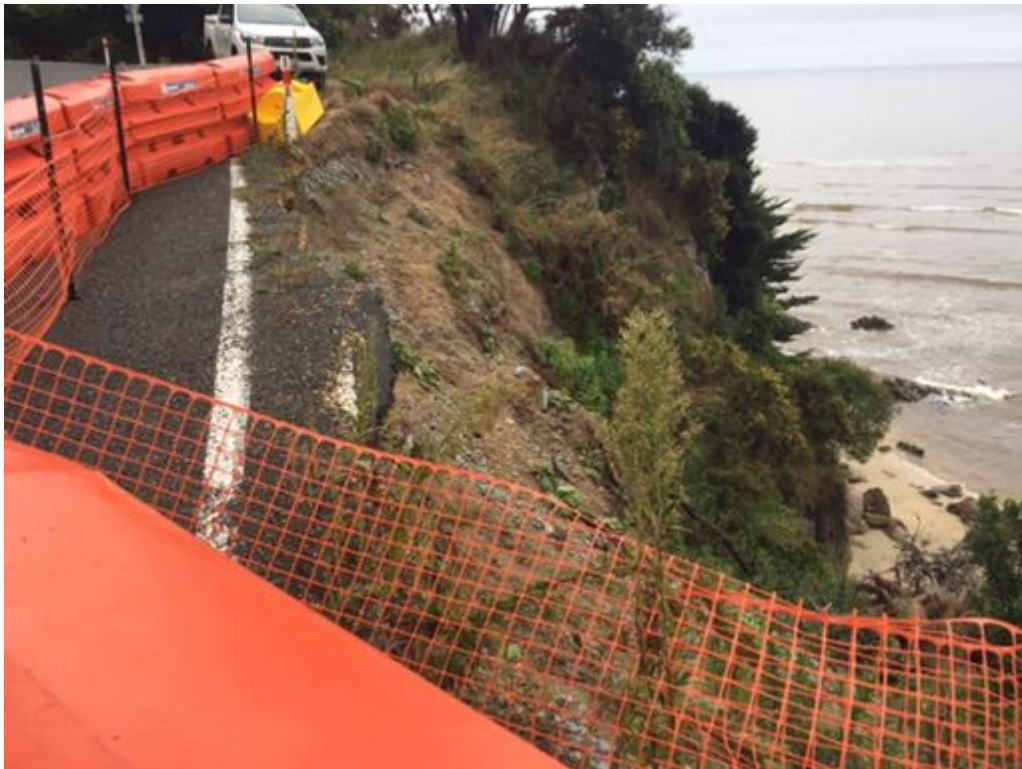
Able Tasman Drive before treatment
