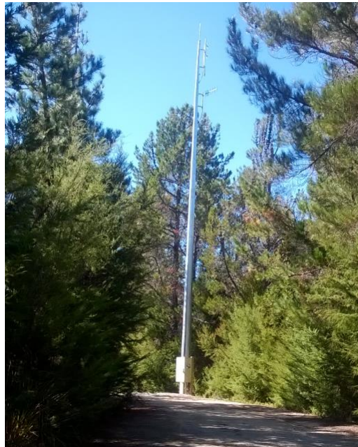
Kaiteriteri SCADA /Telemetry Aerial
