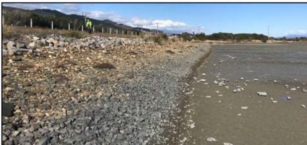
Artificial rip-rap and cobble protection adjacent to the cycle lane and Wakatu Drive.
