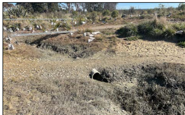
Small pipe and causeway restricting tidal access to upstream salt marsh. Footbridge in background.
