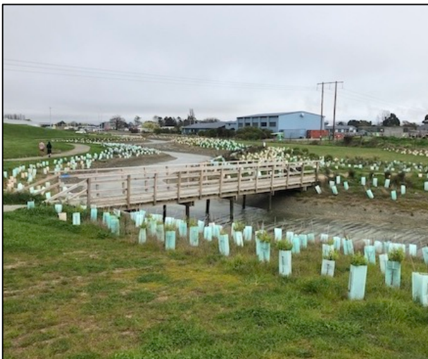
Meanders were built into the lower streamway and the edges reshaped to have a gentle slope prior to planting
