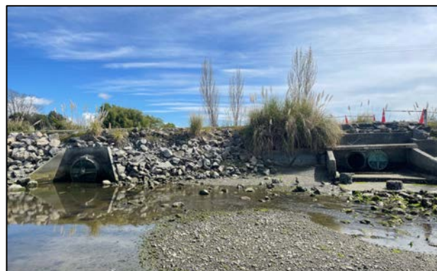
Flapgates on causeway culverts restrict tidal exchange to the embayment (note 2 of 3 flap gates are closed in photo).
