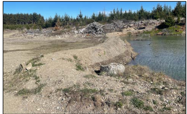
Recently constructed bund at the south of the embayment to prevent tidal inundation of low-lying land.
