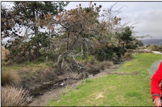
Pine trees growing on an earth bund seaward of a drainage channel running parallel to the shore.
