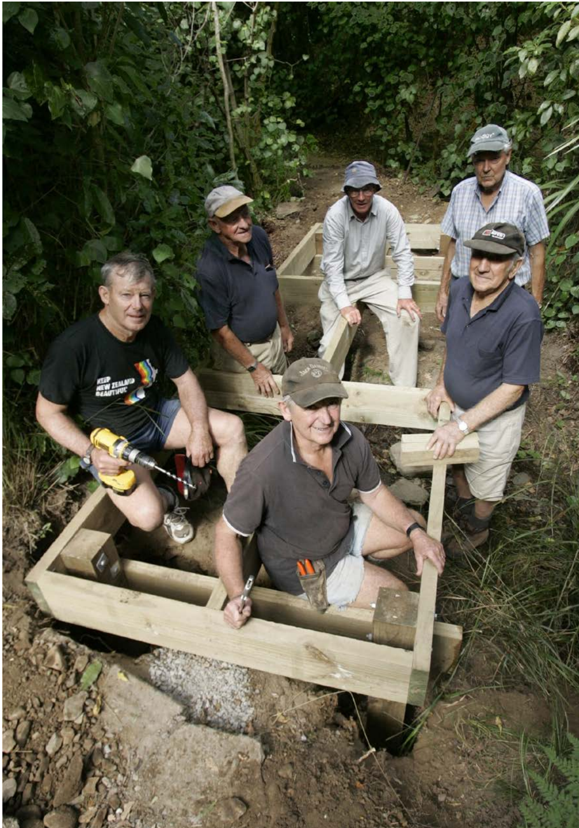
Keep Richmond Beautiful Volunteers constructing a footbridge over Jimmy Lee Creek Walkway, Richmond
