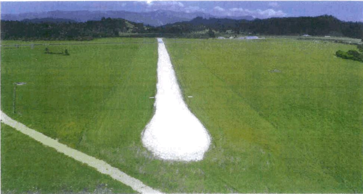
RUNWAY 11/29 THAT REQUIRES SEALING
