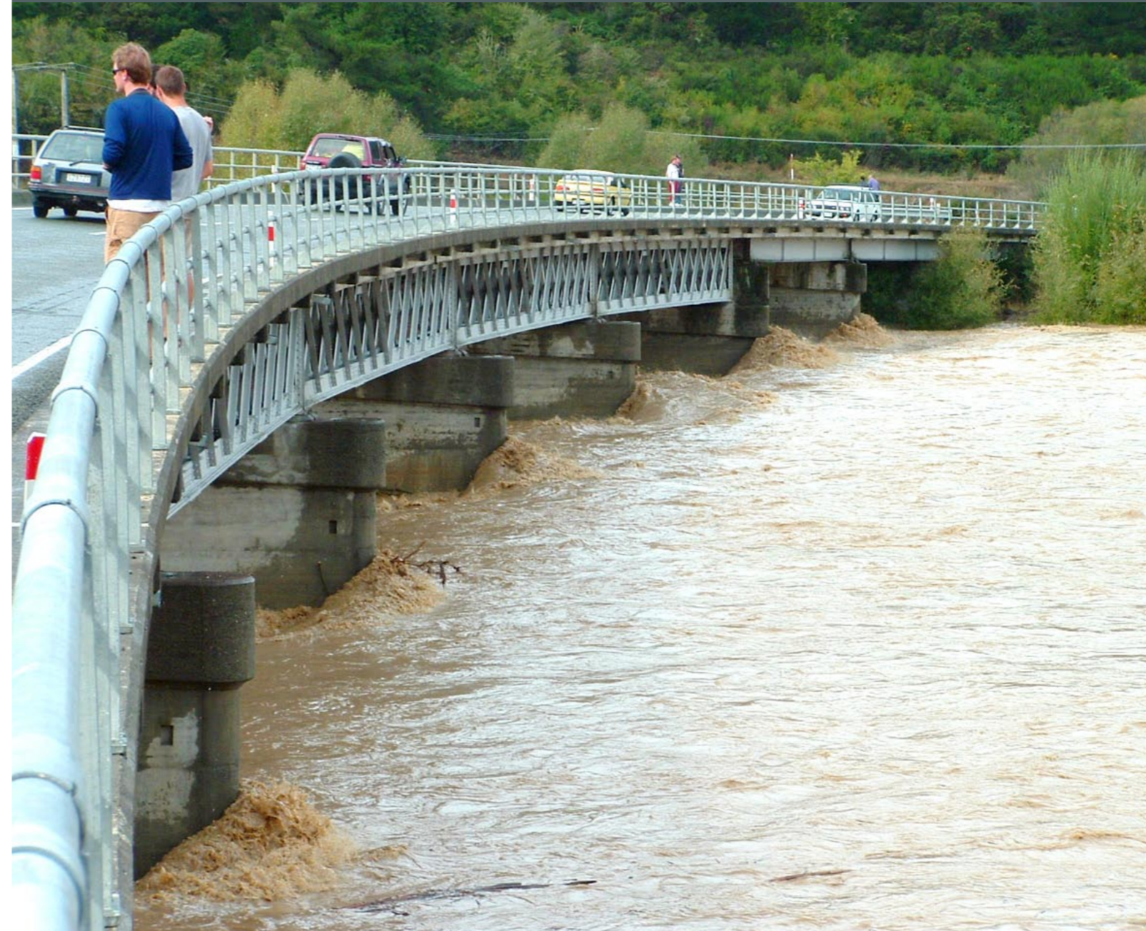
Kohatu Bridge during flood.
