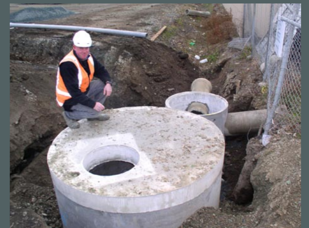
Beach Road humes interceptor.
