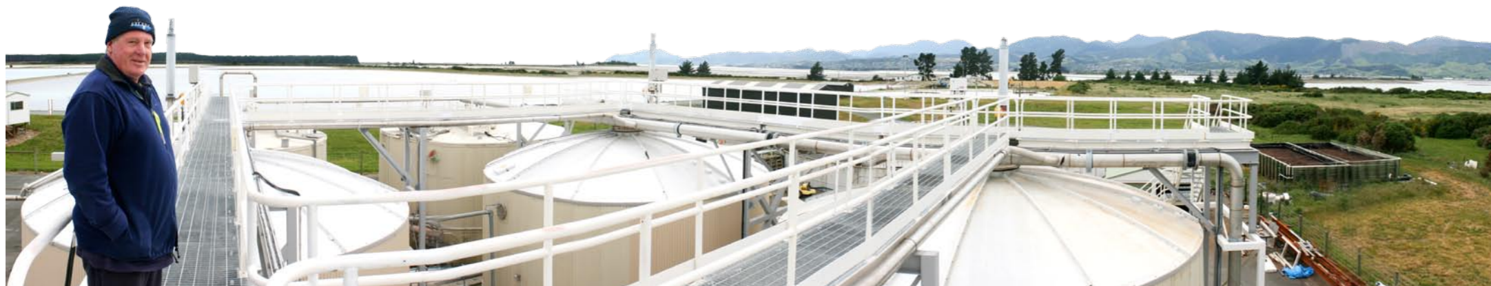
Nelson Regional Sewerage Business Unit facilities at Bells Island.
