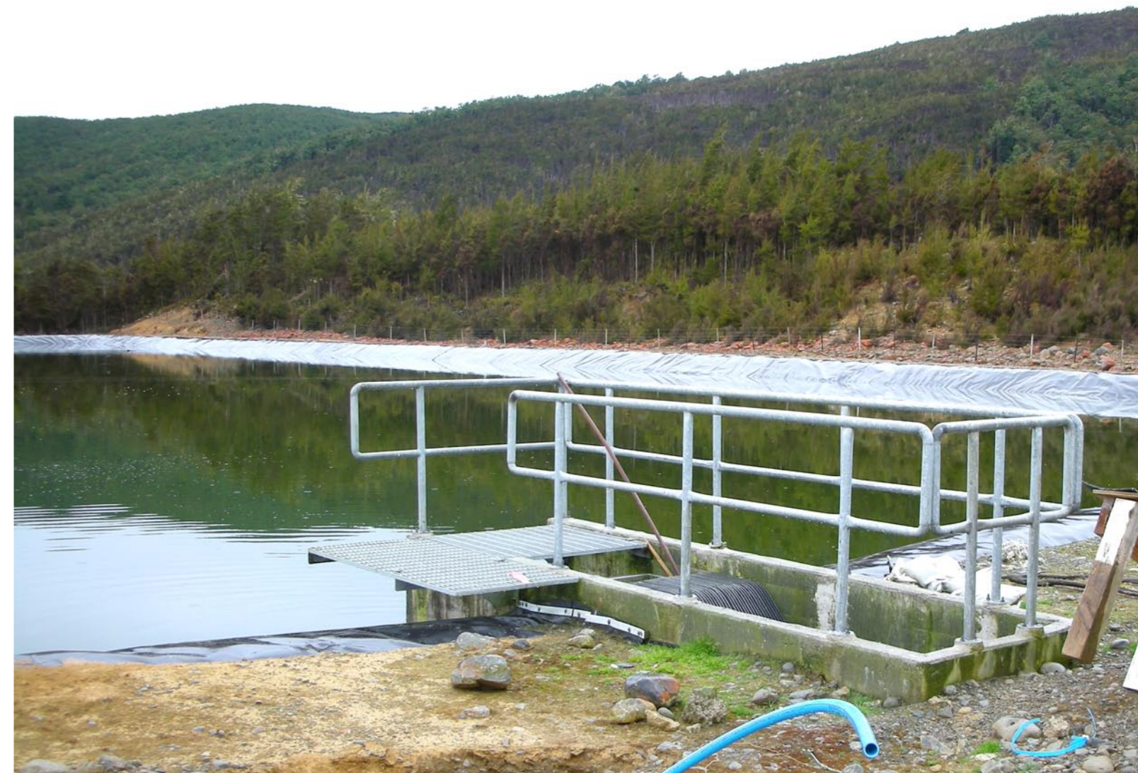
St Arnaud wastewater treatment plant.
