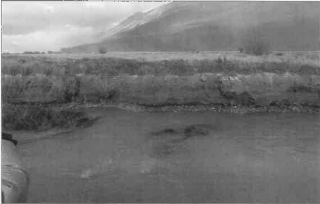
Figure 22 Site 3 right bank following jet boat passage trials (2013 May 25)
