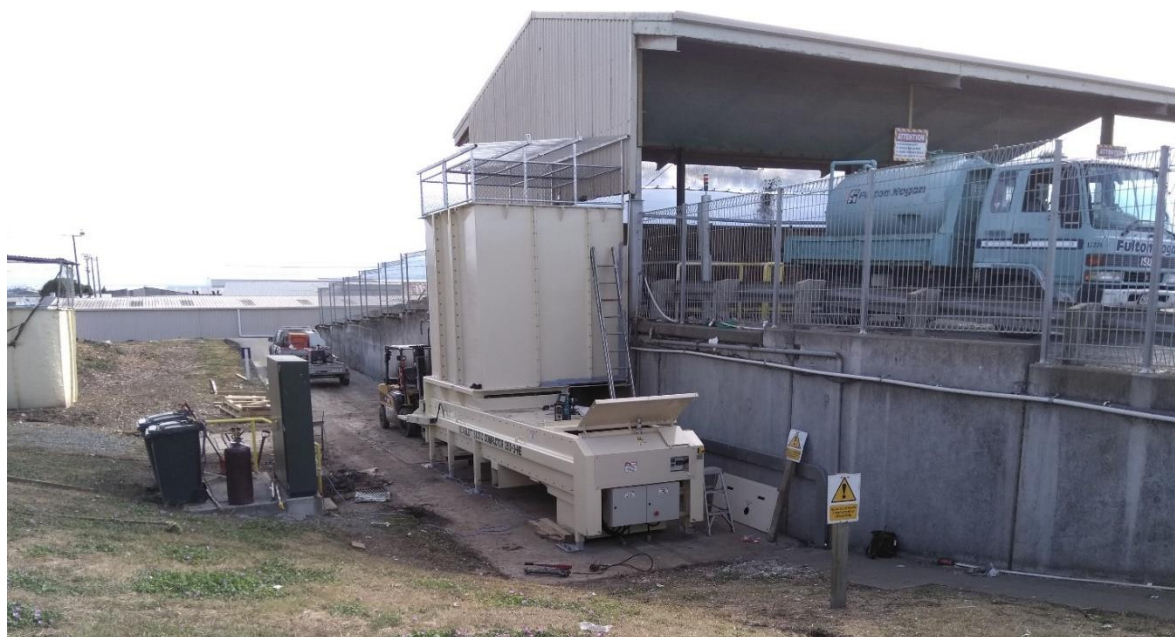
New waste compactor at Richmond Resource Recovery Centre
