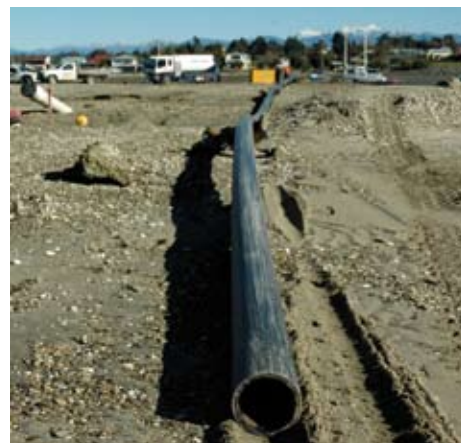
The new sewerage pipe is dragged towards Mapua through an old line.
