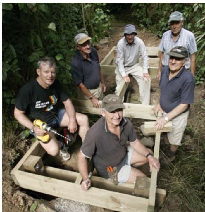
Working on the Jimmy Lee Creek track, from left: Colin Andrews, Larry Norriss, David Burt, Bill Strawbridge, Jack Fearn and Des Henry (front right). Photo: Nelson Mail.
