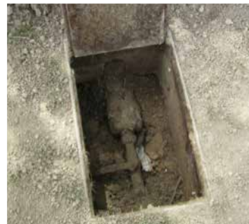
Old water meter
