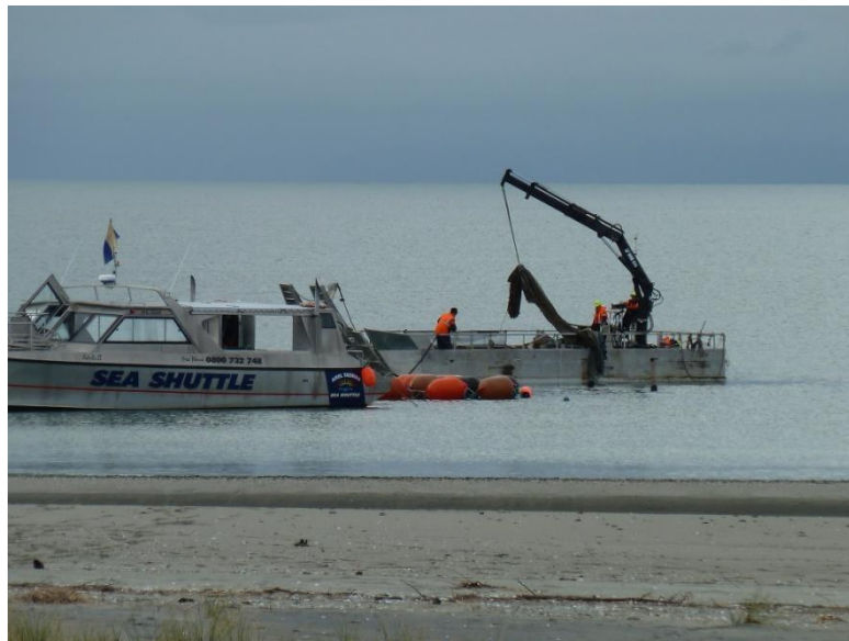
The photographs above show the groyne removal process for the remaining sections under water
