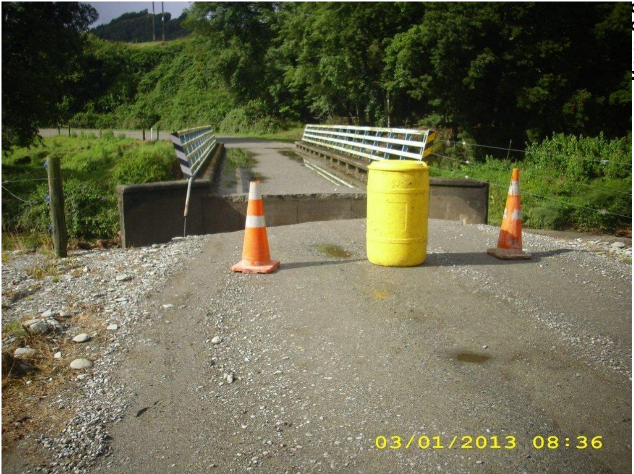
Glenroy Road – Riflemans Bridge approach washed out 3 January 2013
