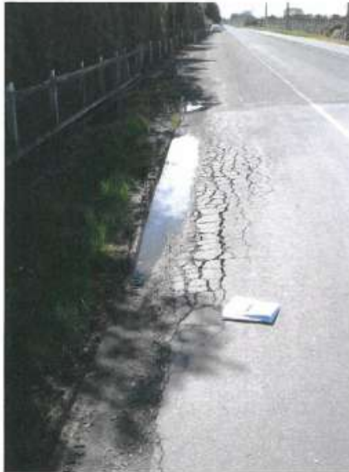
Photo 6: Ponding at Existing Exit to Moutere Highway (north) and associated Pavement Deterioration
