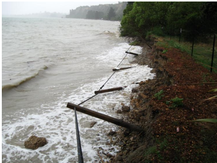
December 2008 Posts and rope falling into the sea
