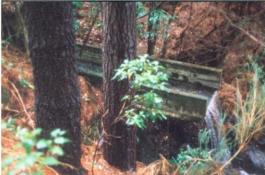
Figure 13: Example of a forestry culvert acting as a barrier to fish passage.
