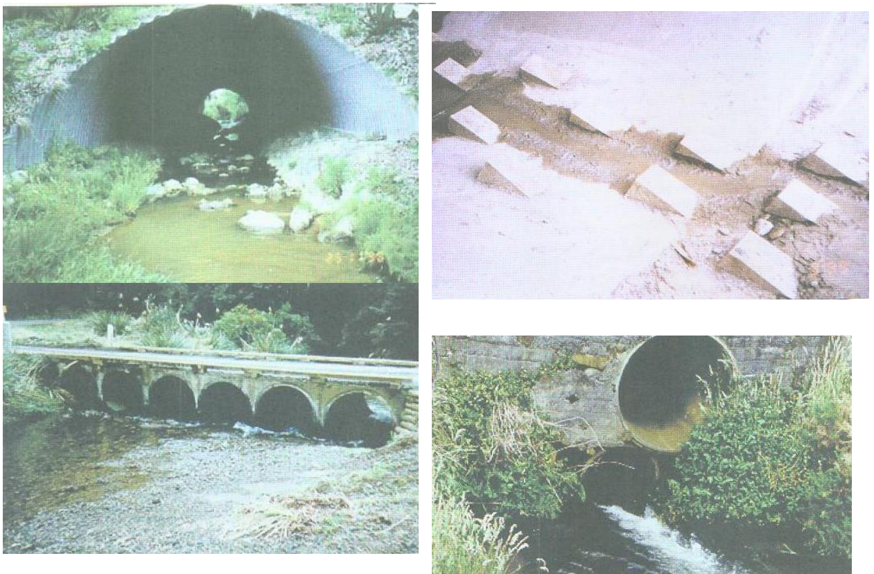
Figure 1; A: Top left: A fish-friendly culvert showing the natural stream bed filling the base.
