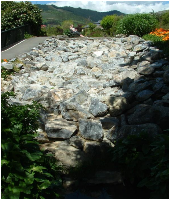
Figure 16: Emergency overflow spillway on Jimmy-Lee Creek at Retention Dam in Washbourne Gardens
