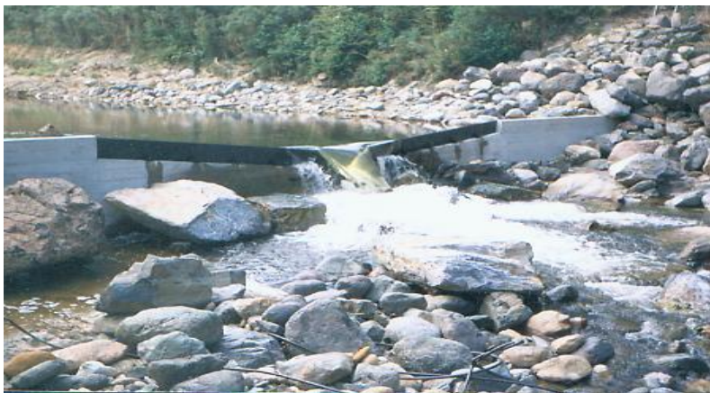
Figure 18: Example of Hydrology Weir at the Maitai River (not in Tasman).
