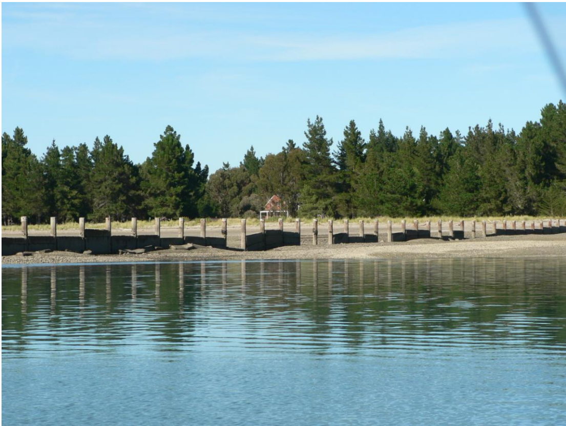
Photograph 2: Existing state of repair of training wall viewed from the channel
