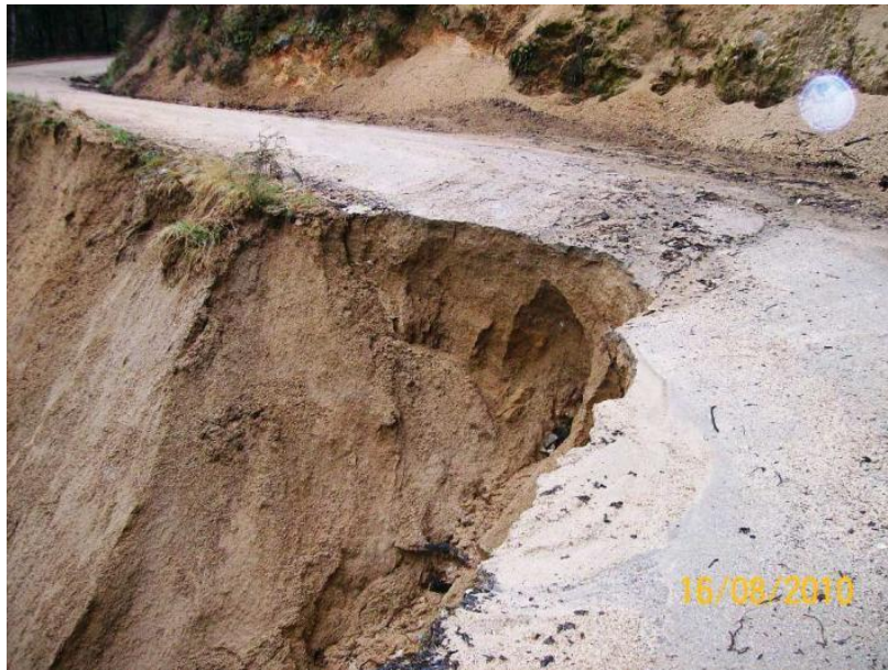
Maruia Saddle Road following slip on 16 August
