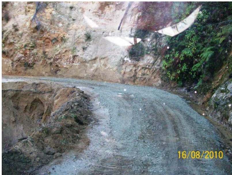
Maruia Saddle Road initial slip response was to bund off face and trim inside of bank to gain width
