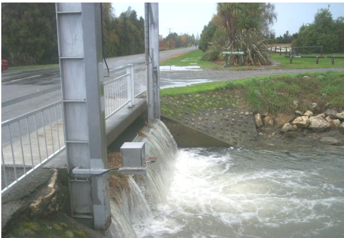
Water Cascading Over Weir with Gates Closed (Note no flooding to Road or Recreation Centre Site Occurred)
